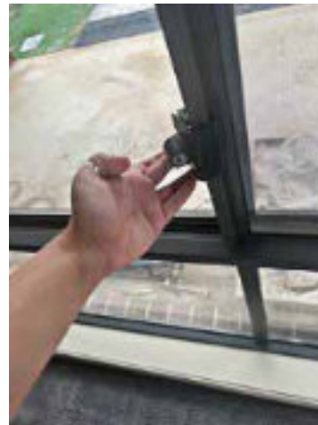
Image 3: broken window lock in Wyndham Vale, presenting a future security issue for a person renting the property.
