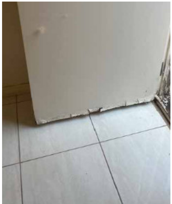
Images 26 and 27: Examples of poor maintenance- a broken light fitting and a damaged door
